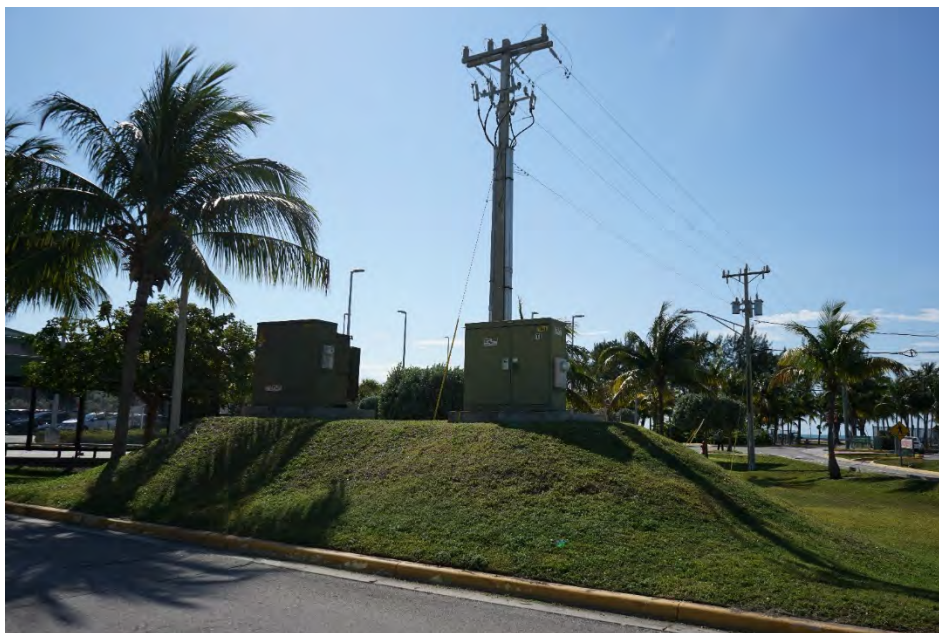
Exhibit 2-35: Main Airport Transformer
