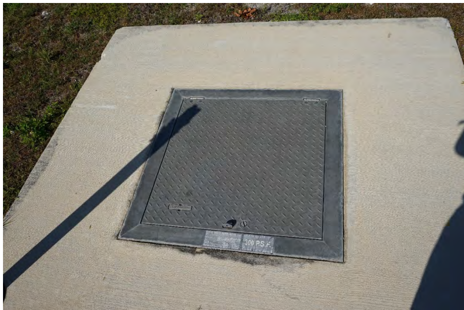
Exhibit 2-36: Injection Well – Access Hatch
